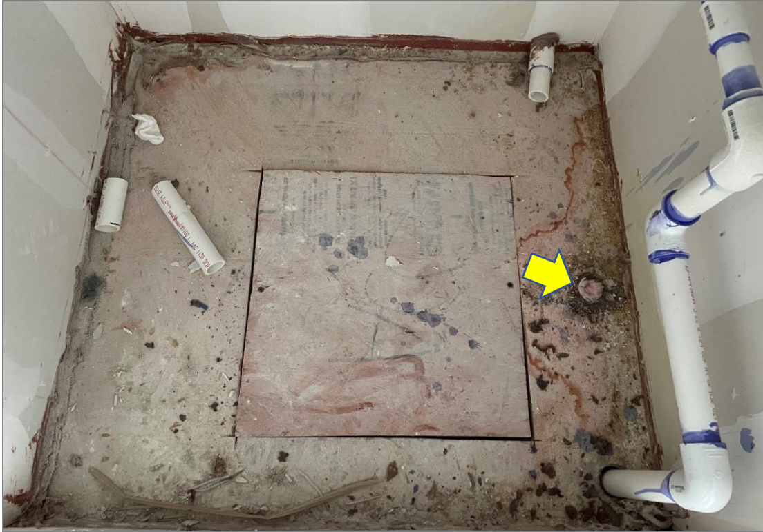
Figure 49. Unsealed condensate access (note relocated drain hole filled with batt insulation).
