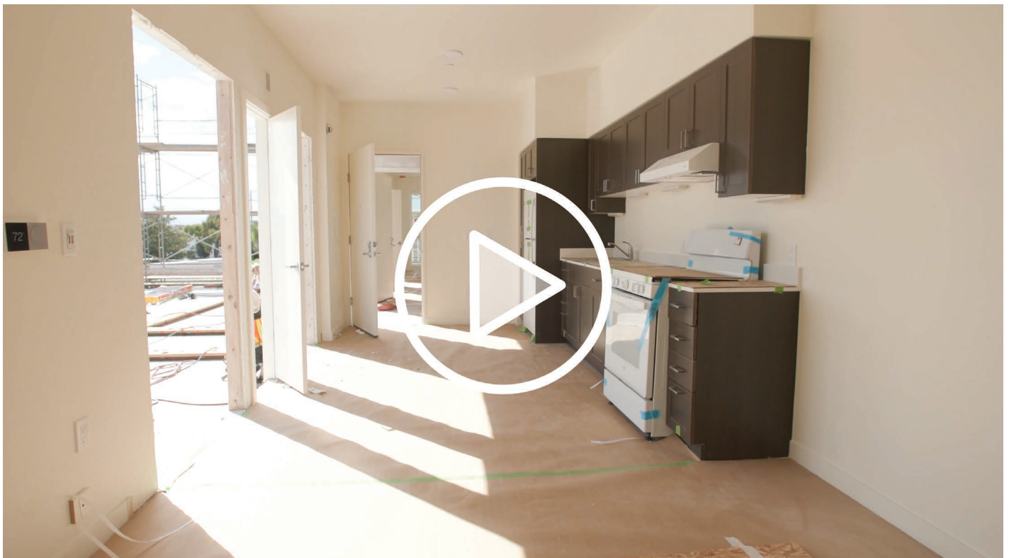
Assembled onsite and up to 80% complete in weeks, the building needs quick protection from rain.
